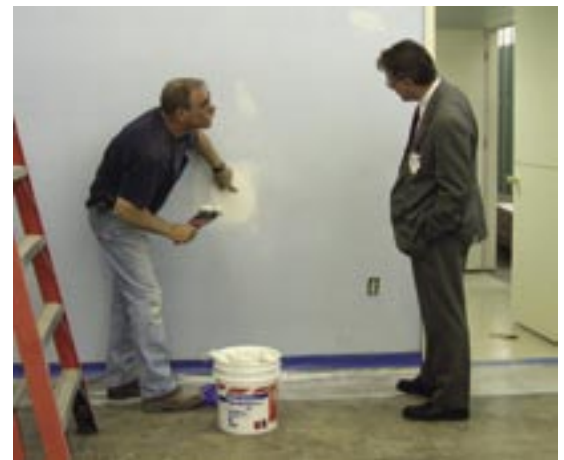
Bruce Phipps, President and CEO of Goodwill Industries of the Valleys, looks over the renovations taking place at Goodwill's Salem facility to accommodate the needs of the collaborative program.
